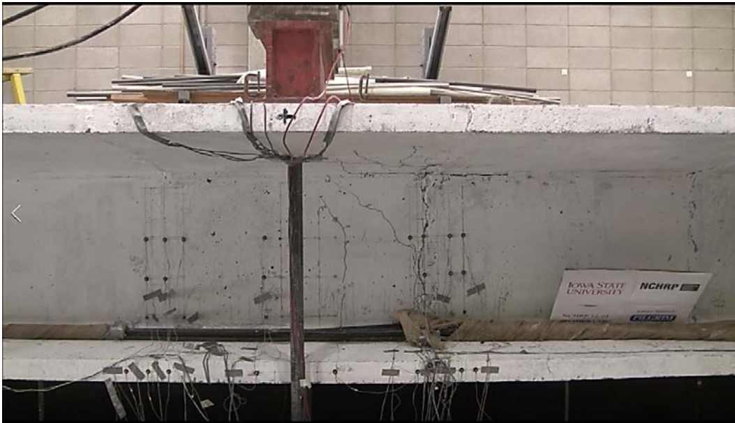
Figure 3.18 – Midspan Condition after Removal of Applied Load to Girder UNB1 after the Test (Sritharan et. al., 2018)
